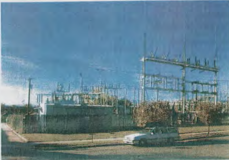
Substation located on 800 South McClelland Street (1054 East)
